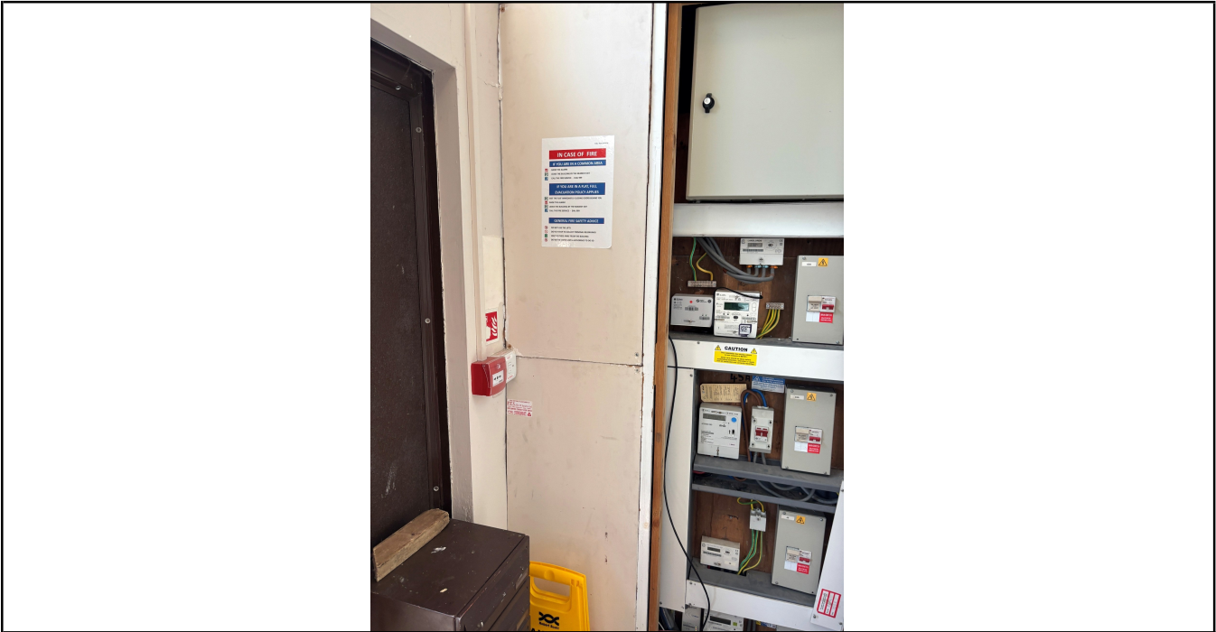
Photo No. 1 Panels replacing service cupboard door,no effective compartmentation
