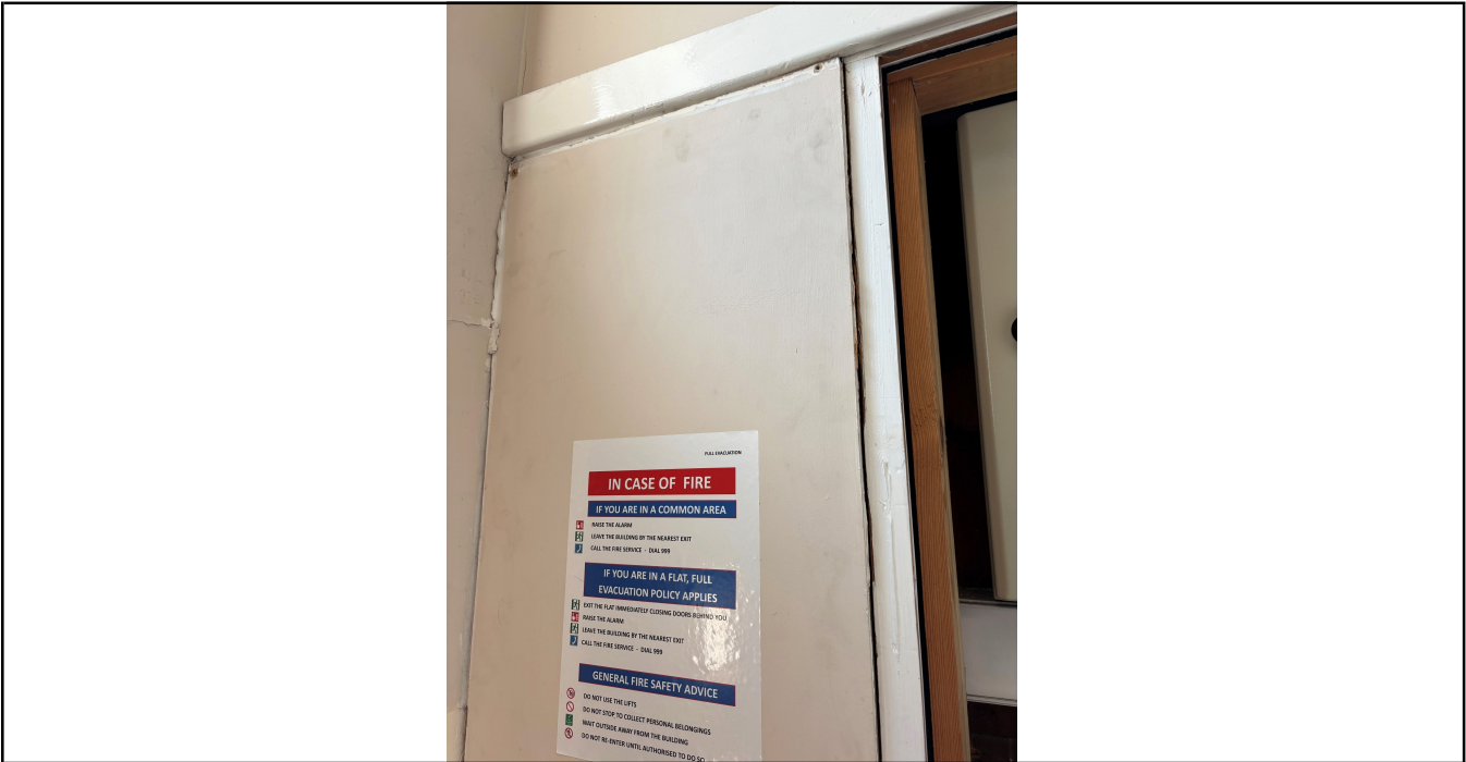
Photo No. 2 Panels replacing service cupboard door,no effective compartmentation
