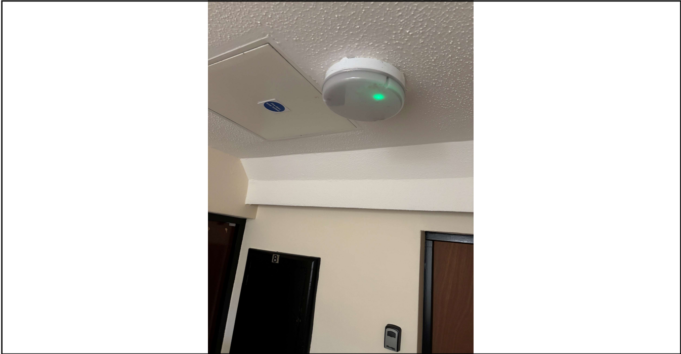
Photo No. 3 One Hour Fire resisting loft hatch and Non maintained mixed system in this block.
