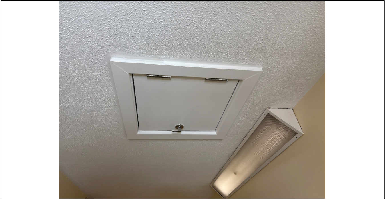
Photo No. 11 Loft hatch has smoke seals but no labelling to indicate fire resistance.
