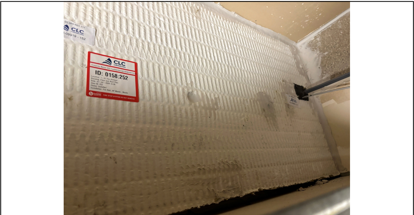
Photo No. 8 Example of fire stopping above cross corridor doors
