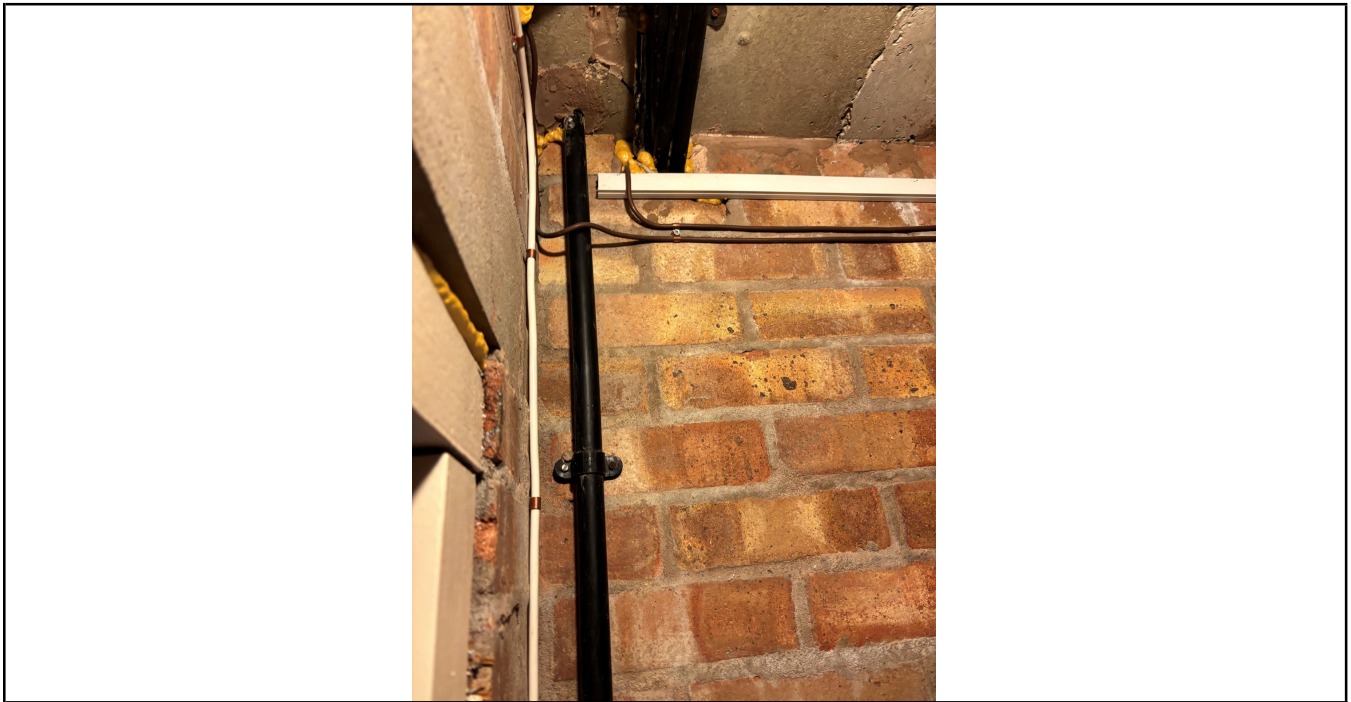
Photo No. 3 Compartmentation breached, Yellow foam use in Electrical room 1stF
