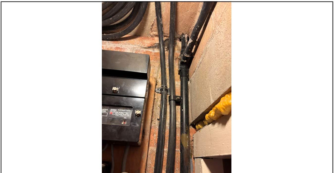
Photo No. 4 Compartmentation breached, Yellow foam use in Electrical room 1stF
