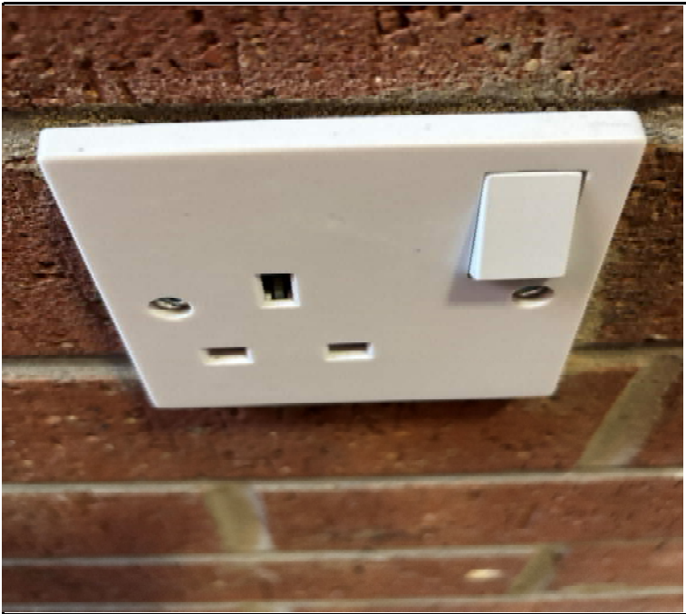
Photo No. 2 Electrical fittings in good condition
