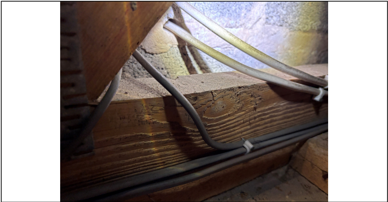
Photo No. 1 Cables breaching compartmentation in loft space
