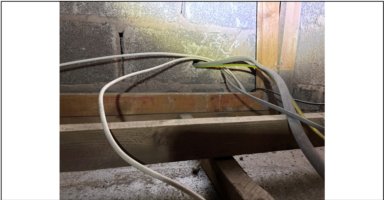
Photo No. 2 Cables breaching compartmentation in loft space
