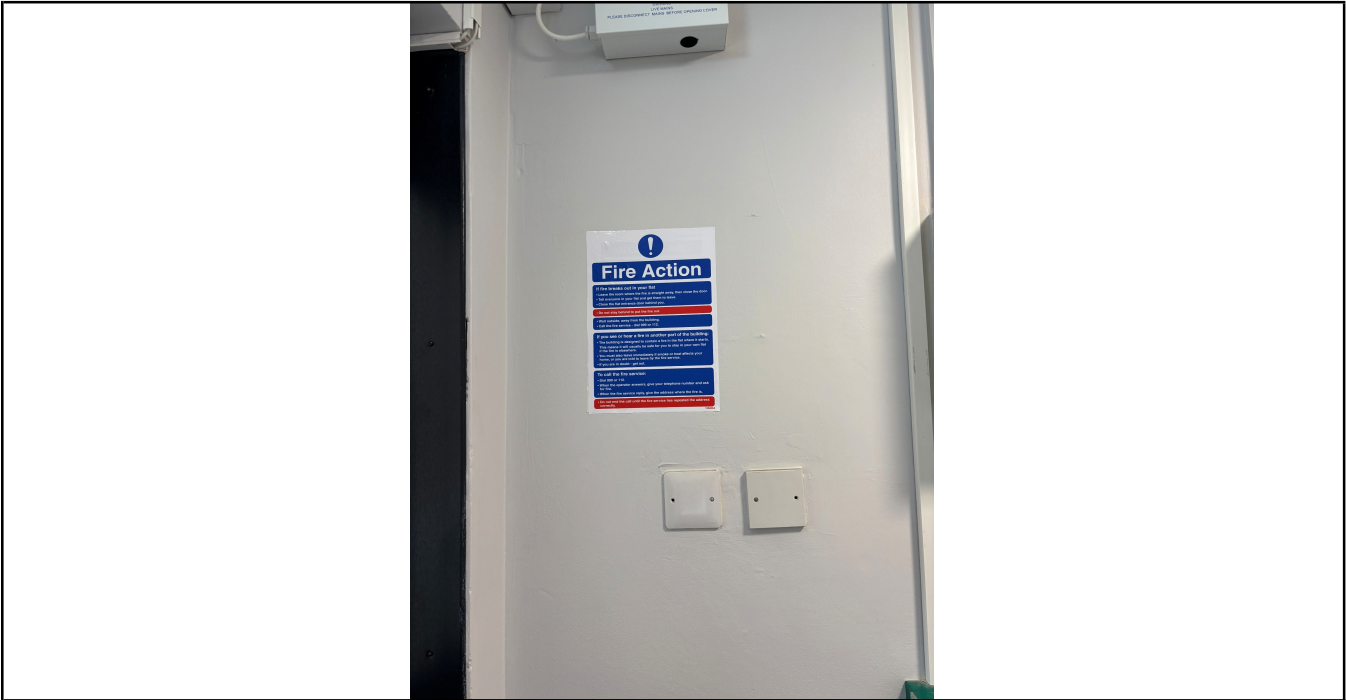
Photo No. 7 New evacuation notices installed
