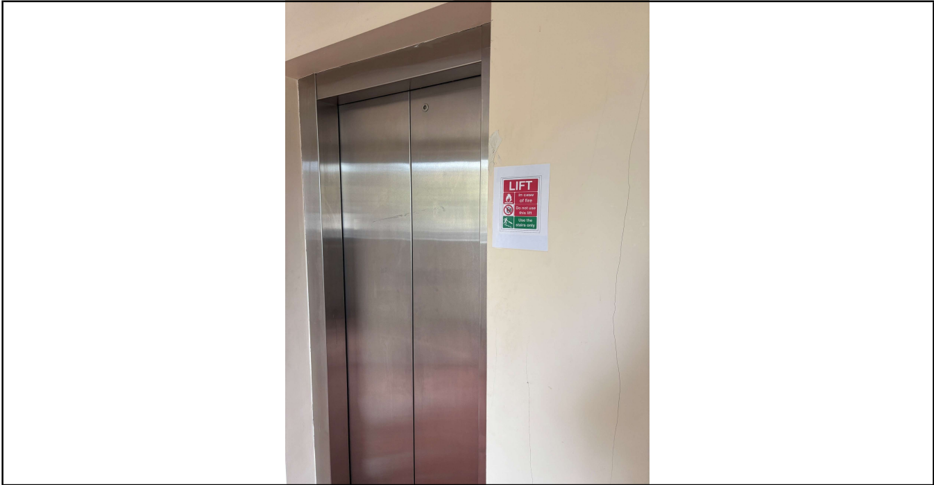
Photo No. 5 Lift Signage
