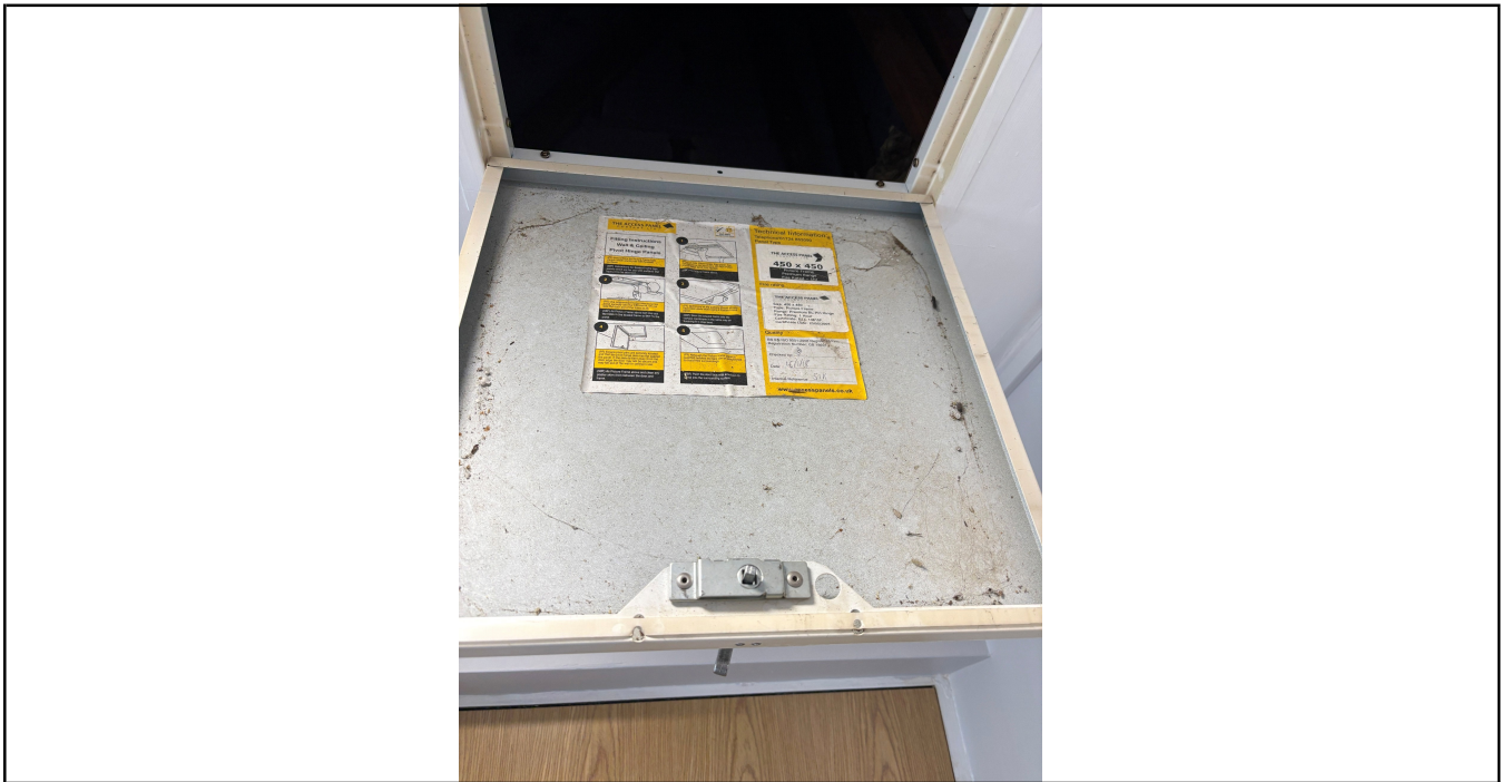
Photo No. 4 1 hr Fire rated loft hatches
