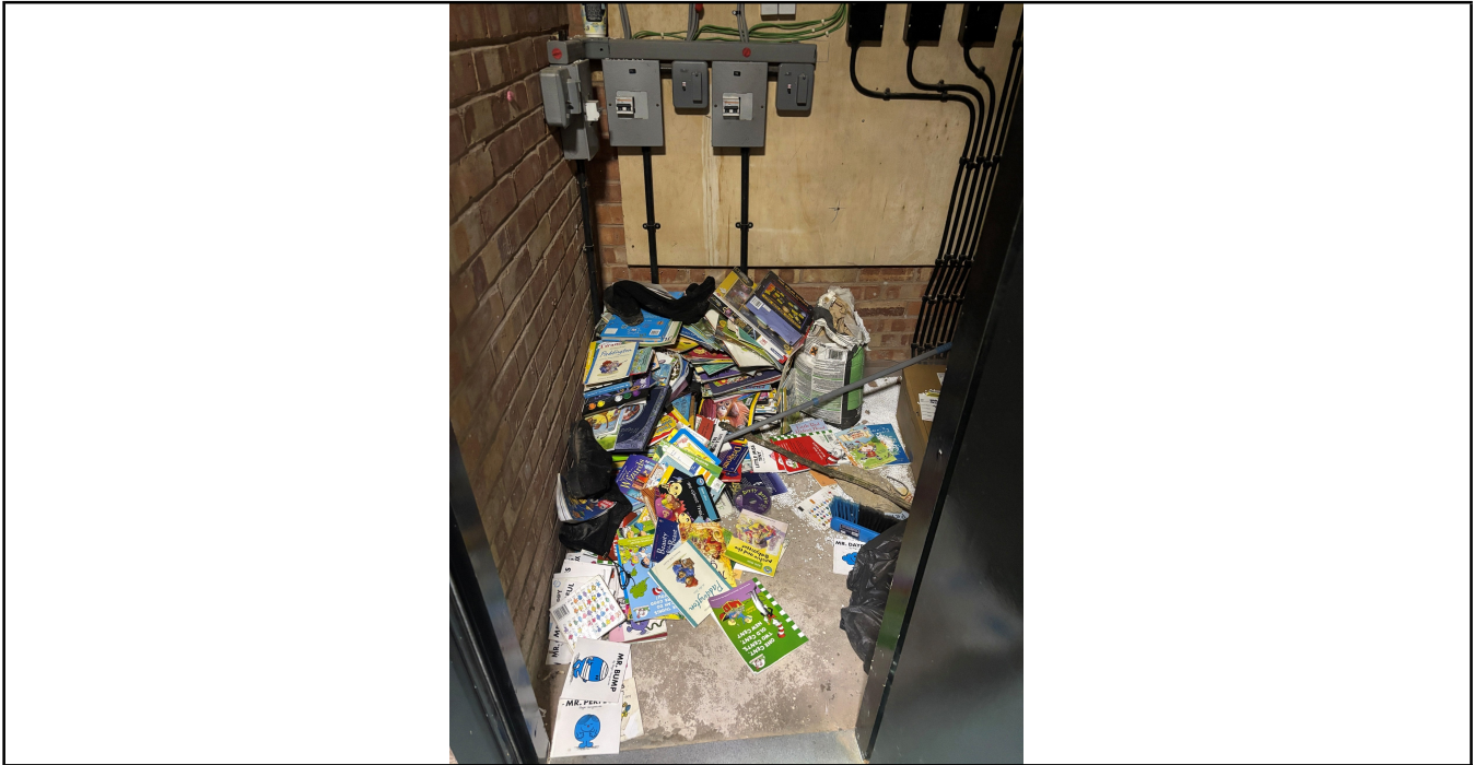
Photo No. 5 Items to be removed from electric cupboard opposite flat 71
