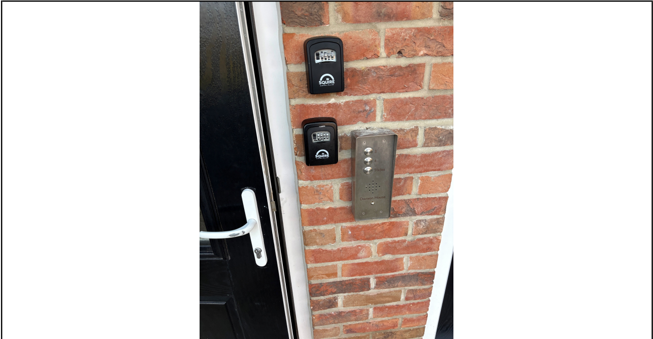
Photo No. 1 Electronic door entry system in place for security reasons.
