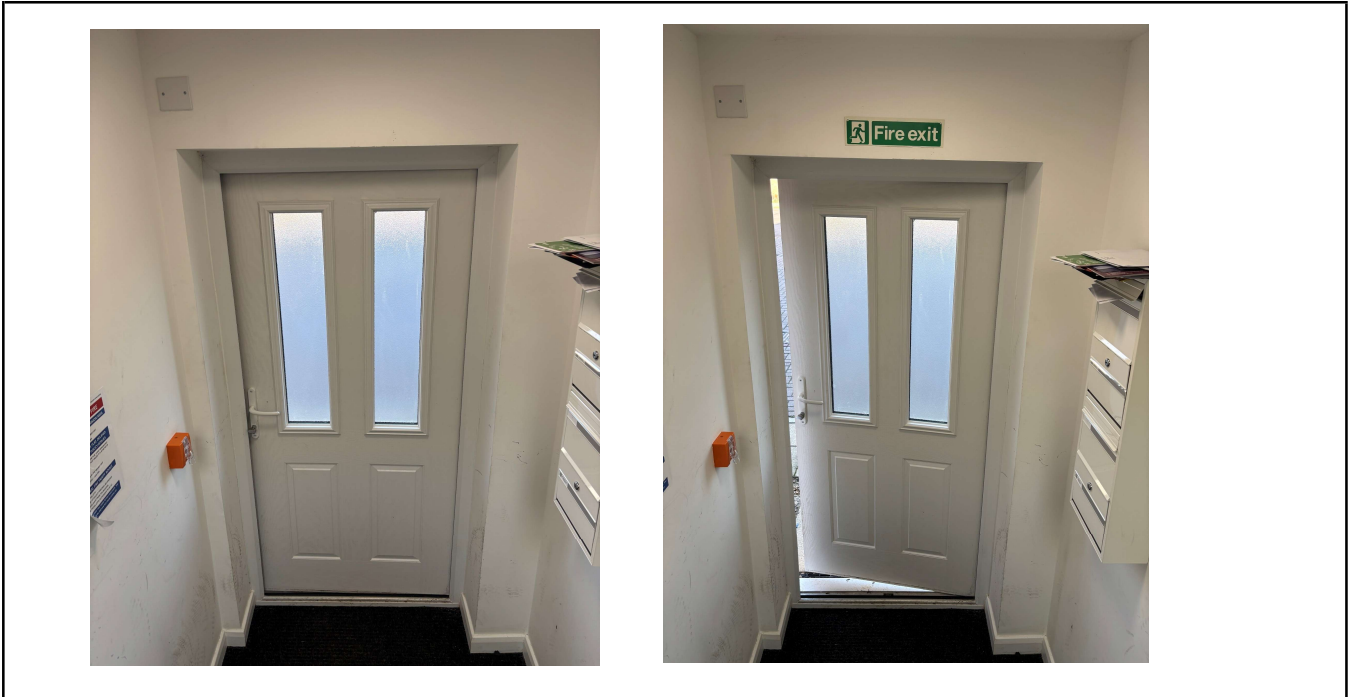
Photo No. 5 Fire Safety action signs updated during the audit.
