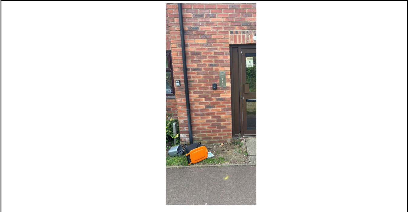
Photo No. 1 Electronic door entry system in place.
