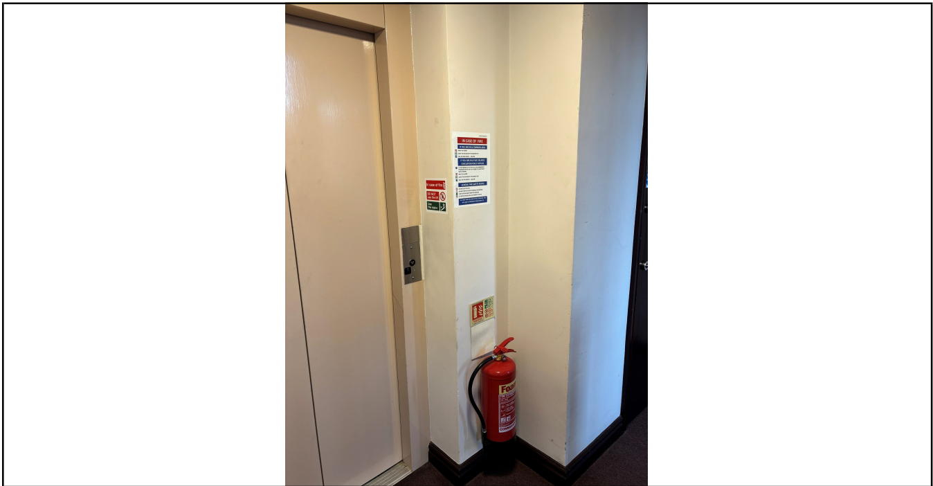
Photo No. 6 Lift and Evacuation notices in place
