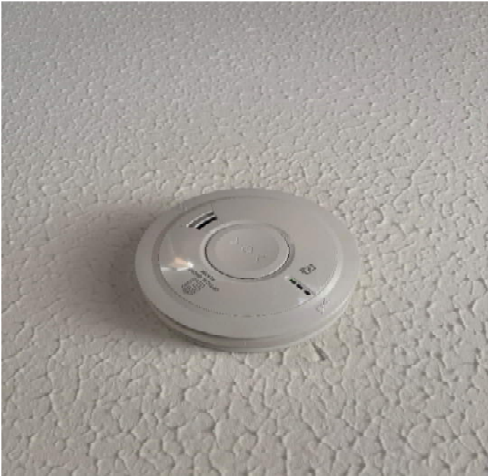
Photo No. 1 Fire detection fitted and in good condition
