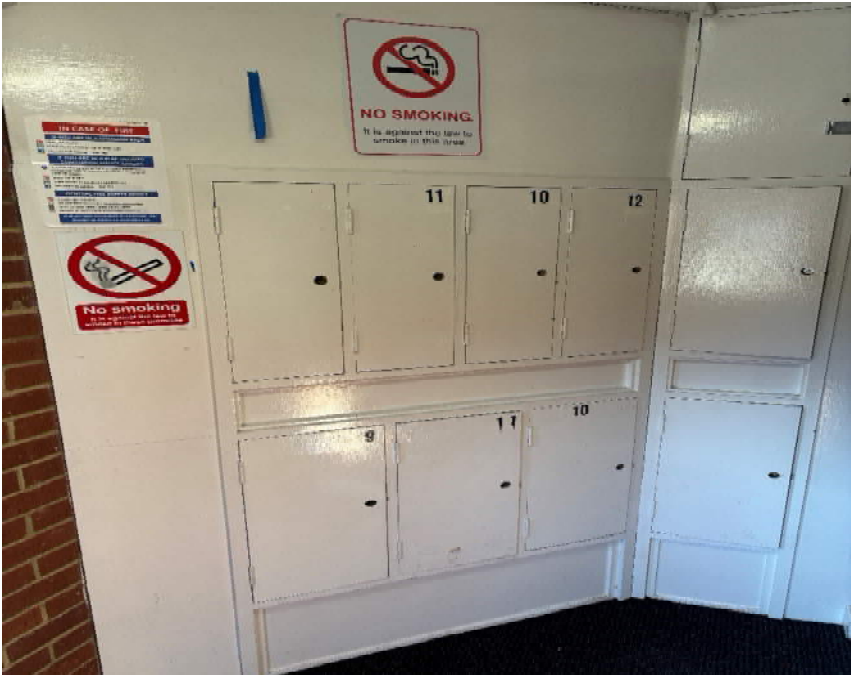
Photo No. 2 Electrical and Gas intake cupboards with correct signage displayed
