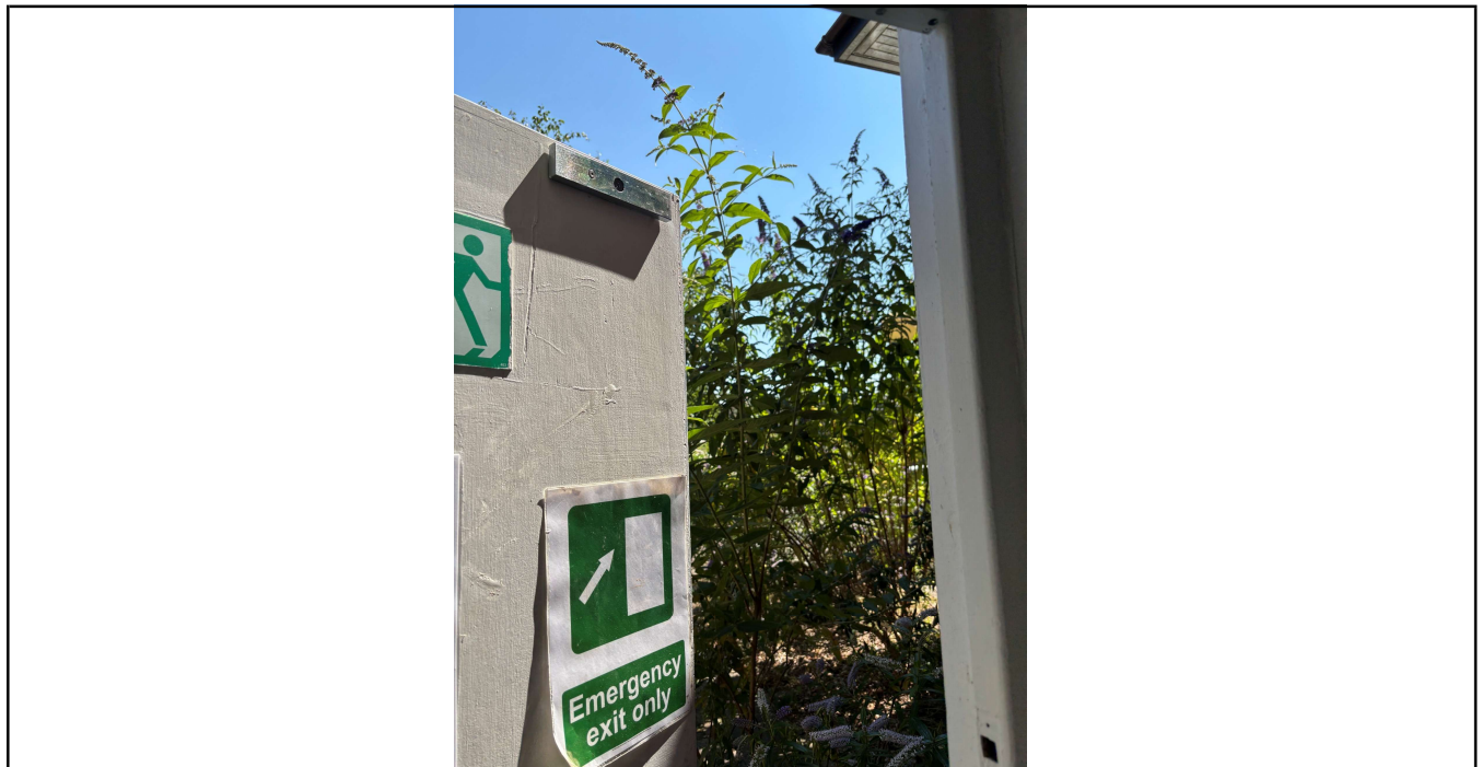
Photo No. 5 Mag locks on exit doors releasing on fire alarm activation
